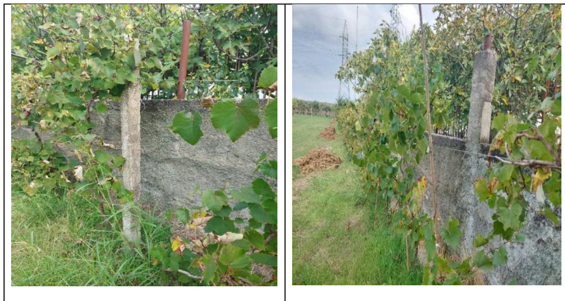
Figure 18 Affected fence wall in TPS Sallmone
