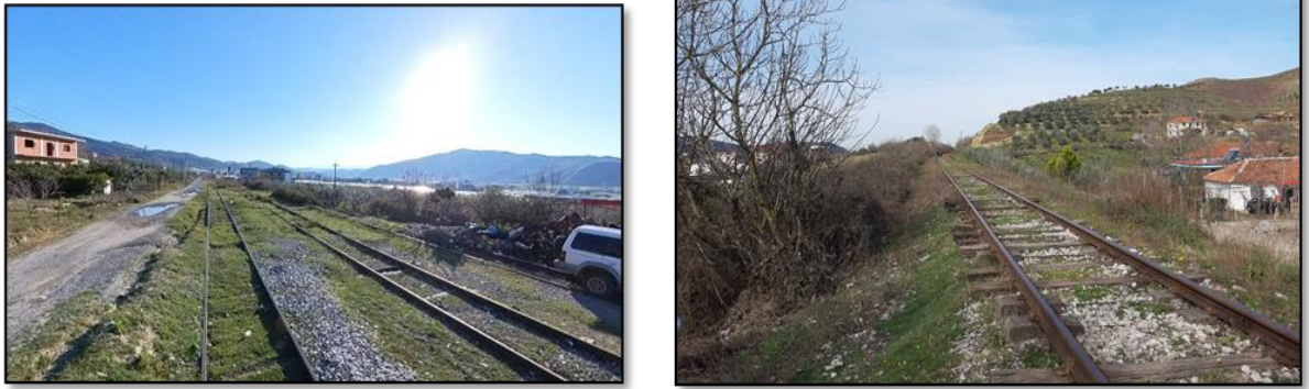
Figure 2-2: Infrastructure condition of the railway line between Rrogozhinë and Elbasan
